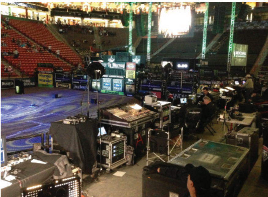
Figure 5. Fiber cable with a rigid central strength member is of vital importance in permanent installations. Fiber cable is pulled through conduit and is often exposed to 10 times the tension it would normally incur.
